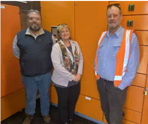
Silas Darby, Jackie Kruger and Chris Dole reviewing the electrical upgrades at the Leeton Sewage Treatment Plant
