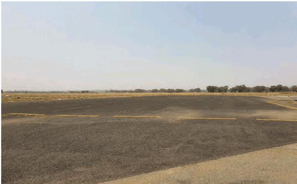
Fig 3 – The current available AAPA parking apron as viewed from adjacent the refueling point. While not shown in the photo, the apron is floodlit.
