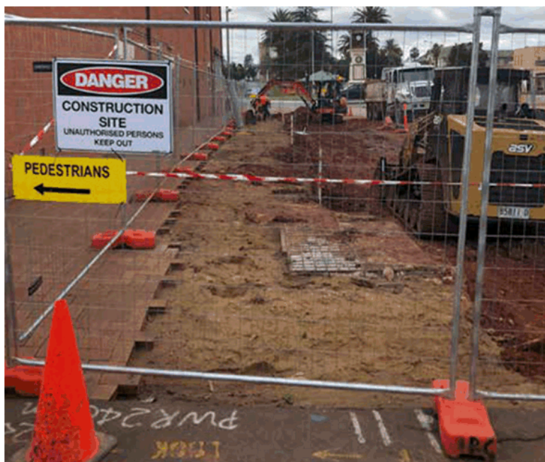
Works in progress in Wade Avenue. Our WHS training helps to keep our worksites safe for our staff and the community
